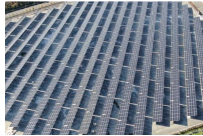
Shiga-Takatsuki Plant solar power system
